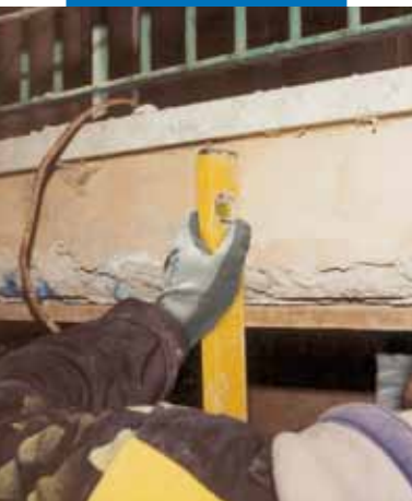
Restoring the front of the concrete slab of a balcony: positioning wooden form work
